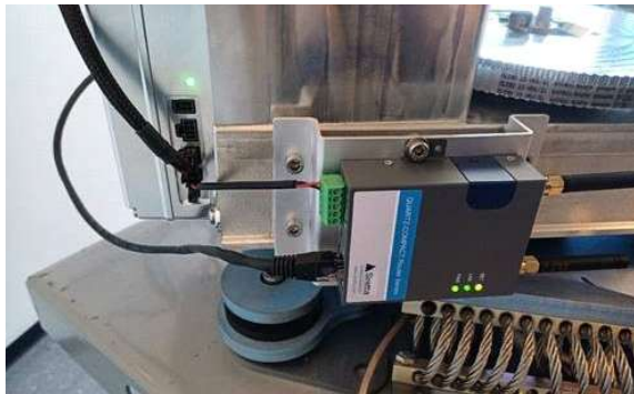
Figure 2-39: LTE modem connection, example
