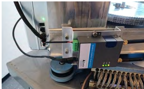
Figure 2-24: LTE modem connection, example
