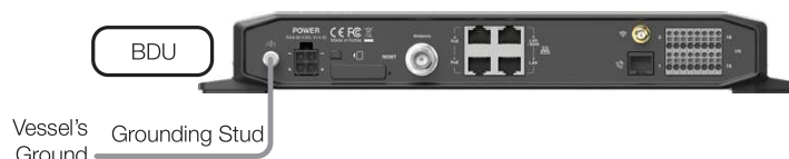
Figure 38: Grounding Stud Connection
